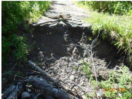
Washout prior to repair
